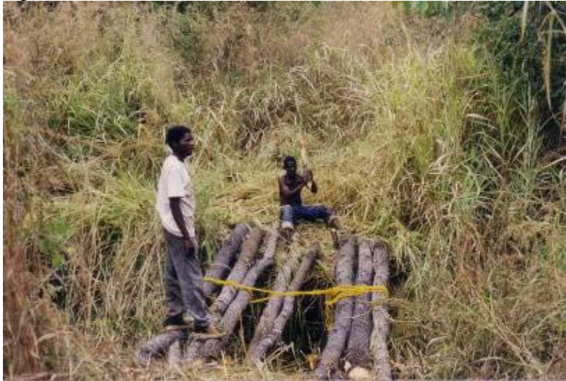
Constructing Road to Paulila (1998 and then 1999) – Caetano Tuli (right) and District Agricultural Officer
